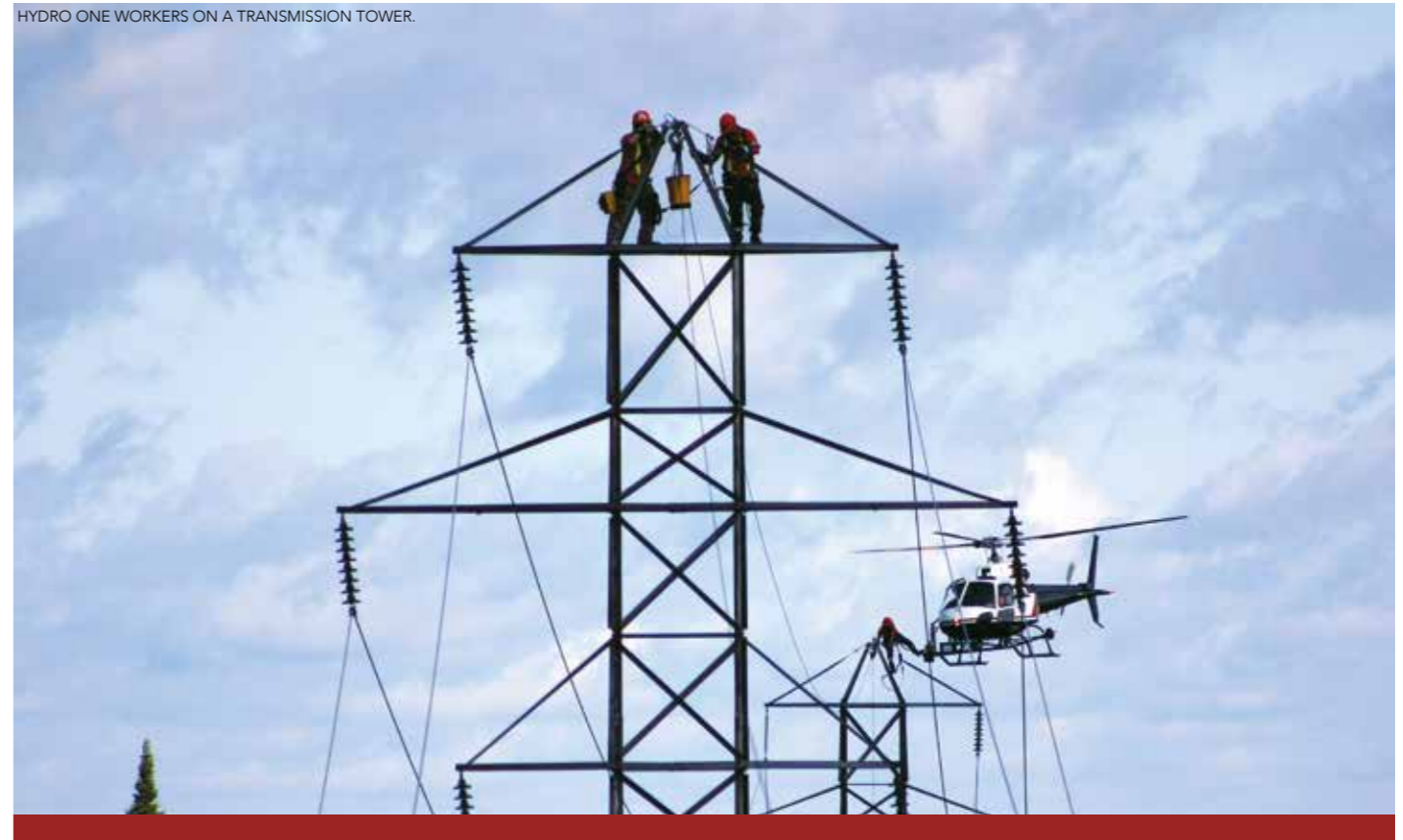
HYDRO ONE WORKERS ON A TRANSMISSION TOWER.
