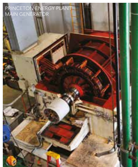
PRINCETON ENERGY PLANT POWER TURBINE
