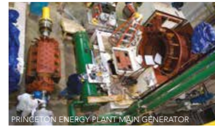
PRINCETON ENERGY PLANT MAIN GENERATOR
