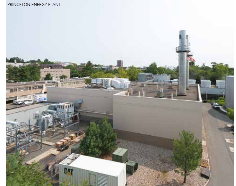
PRINCETON ENERGY PLANT
